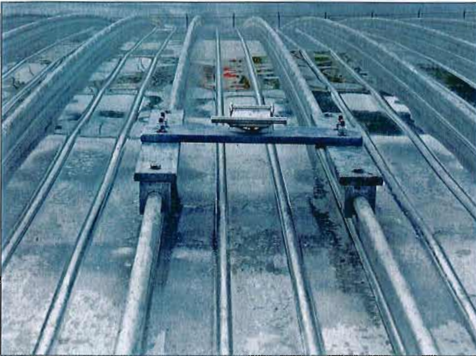
Photo 3 – Example of anchorage points with horizontal lifeline installed on a standing-seam metal roof at Northwest Florida Beaches International Airport. Illustrates plan point of view similar to configuration depicted in Figure 2. System is designed for fall-arrest requirements only. Photograph courtesy of Pro-Bel.
